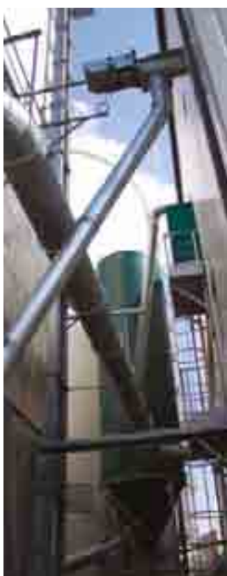
CHP plant, Belgium
