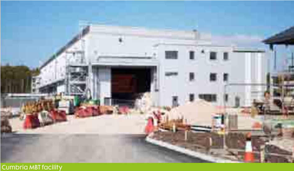
Cumbria MBT facility
