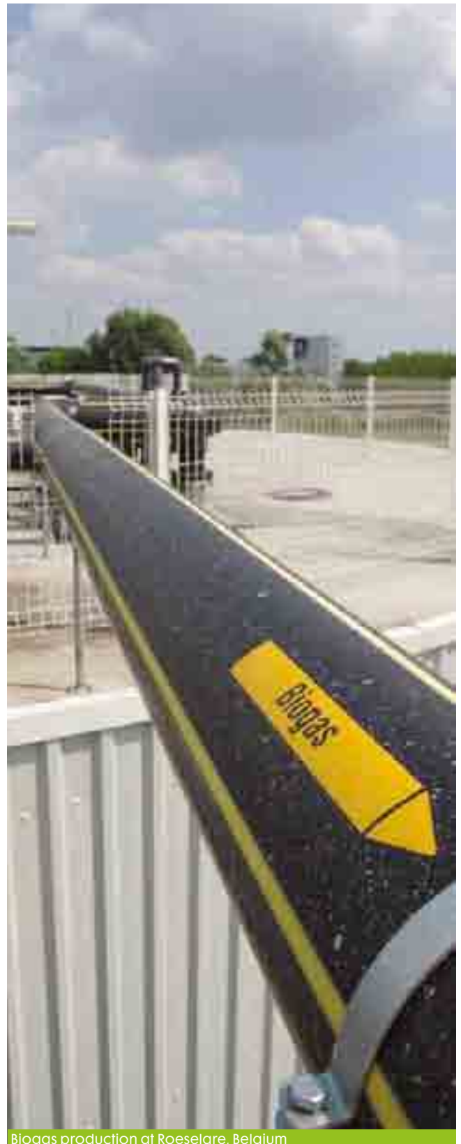
Biogas production at Roeselare, Belgium
