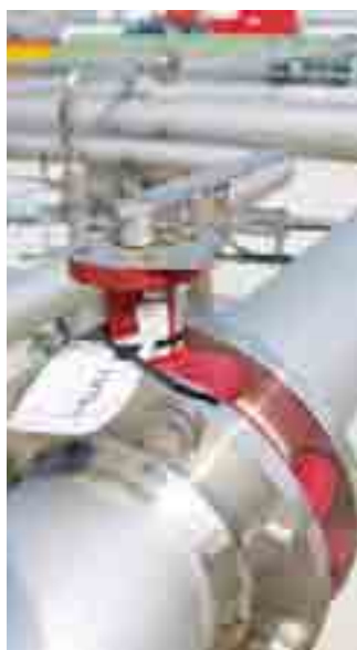
Greenmills AD Facility
