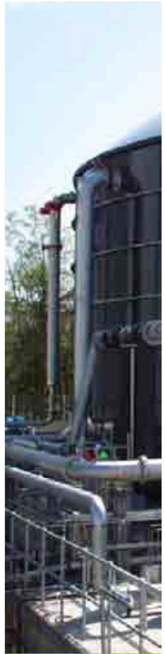
Cumbernauld AD facility
