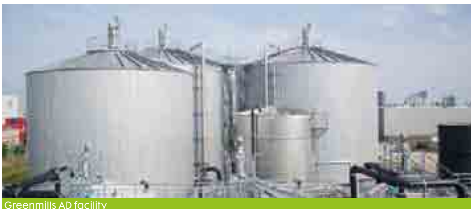
Greenmills AD facility
