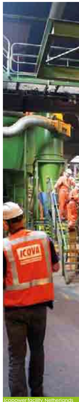
Icopower facility, Netherlands
