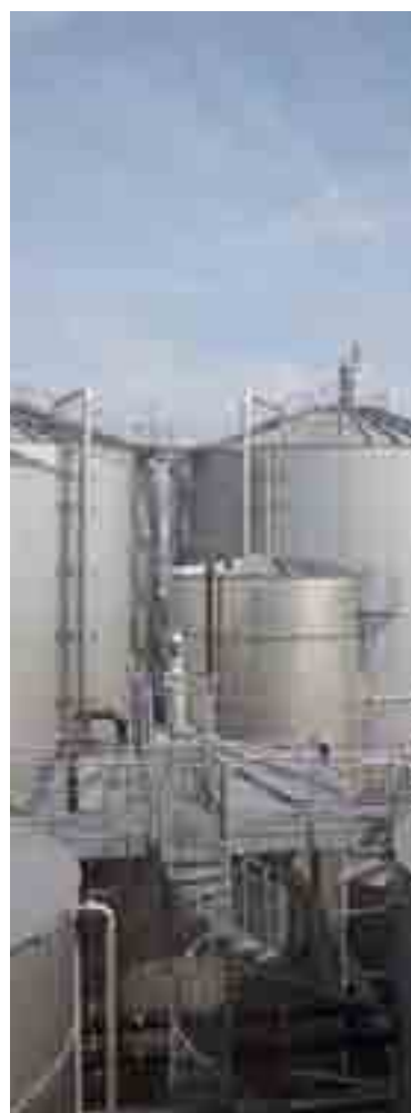
Greenmills AD facility, Netherlands
