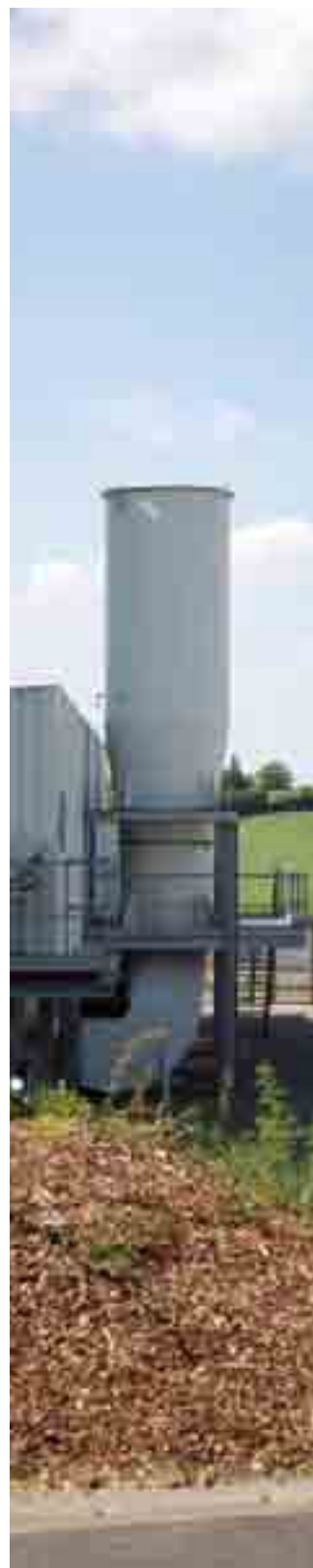
CHP plant in Belgium
